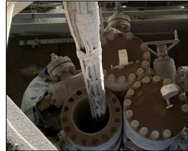
Well configuration at surface
