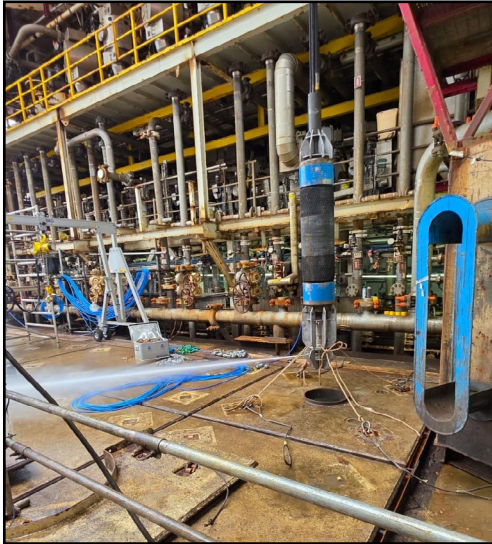
xcalibre System Test before deployment
